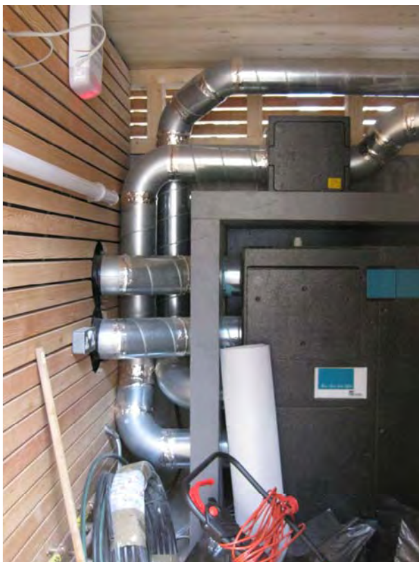
Figure 2-6. Heat Recovery Ventilation unit (BEFORE DUCTWORK WAS INSULATED) inside the frost-protected unit in the external bike shed.
