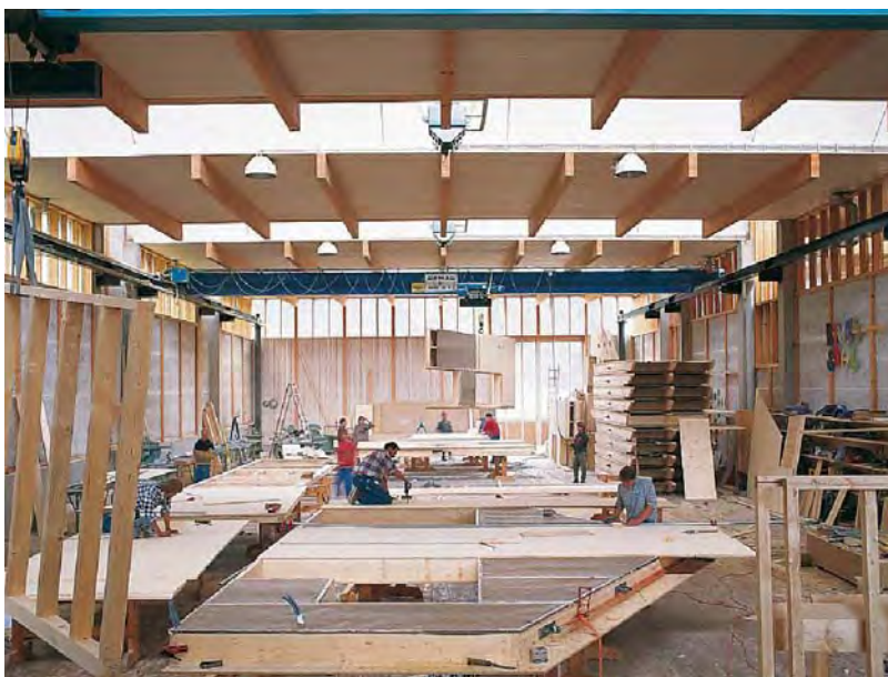
Figure 2-8. The timber frame was prefabricated in Austria by Kaufmann Zimmerei of Reuthe
