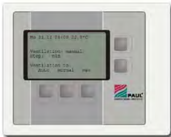
Figure 2-7. Ventilation control installed in the living room
